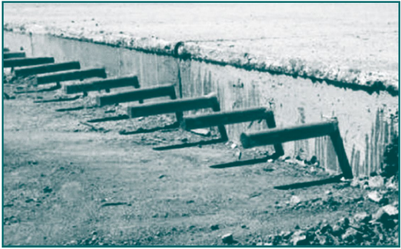
Figure 5. Photo of epoxy-coated dowel bars in full-depth concrete pavement repair (photo credit: www.pavement interactive.org)
