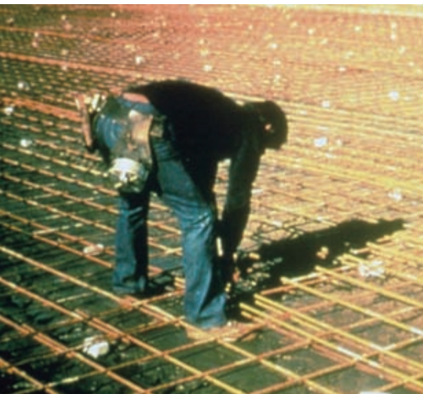
Heavy continuous reinforcing to eliminate contraction joints and only have tight cracks.
