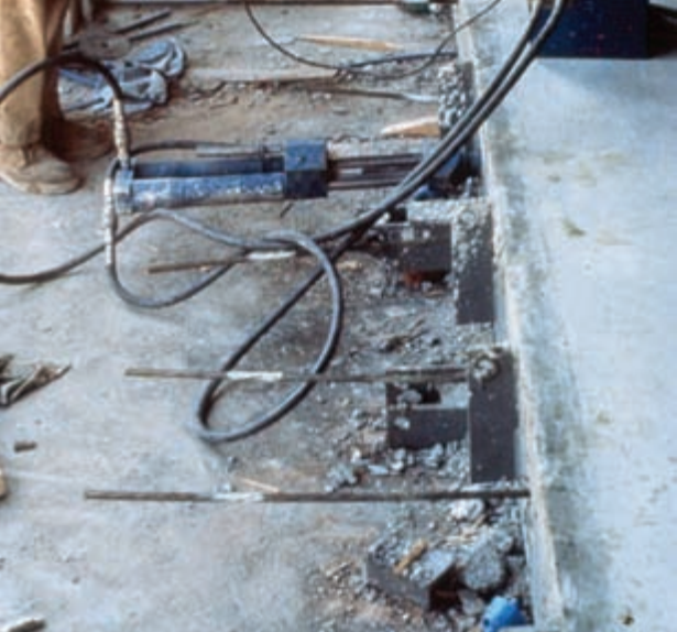
PT jack and tensioned tendon with total elongation of 27 inches. Note white paint marking partial elongation in staged jacking.
