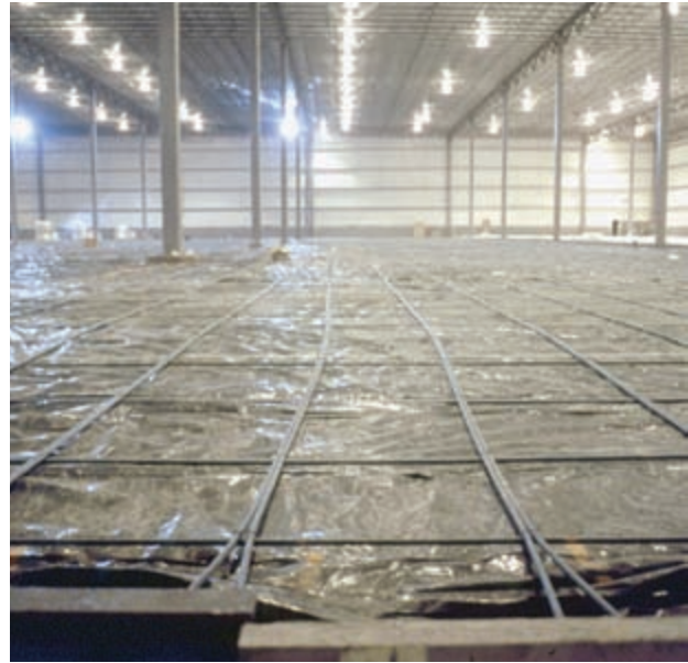
A 340x125-foot distribution center floor slab with two-way bundled PT tendons and no joints or cracks after eight years. Note void former offset so that bollard will be centered after 1 inch plus of slab movement.
