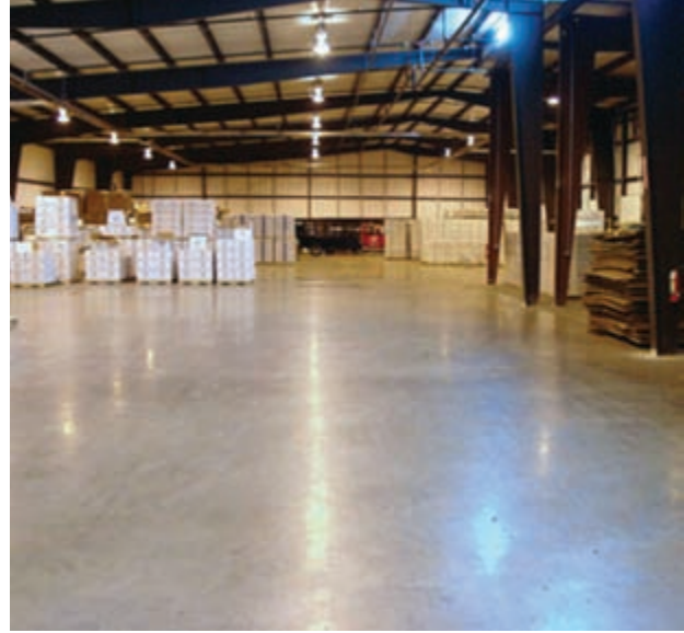
A 127x60 foot warehouse floor slab 6 inches thick with HVSF and no joints or cracks after three and a half years.
