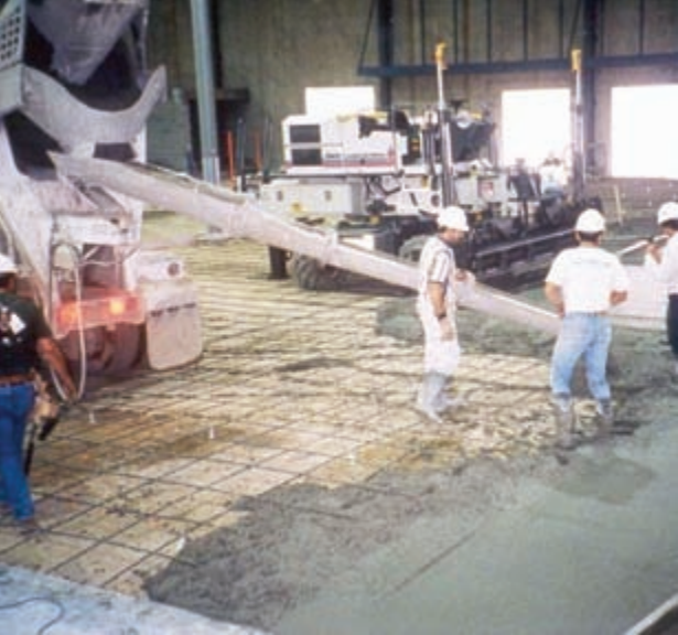
Light reinforcing continued through contraction joints for load transfer and chaired up just before concrete placement.
