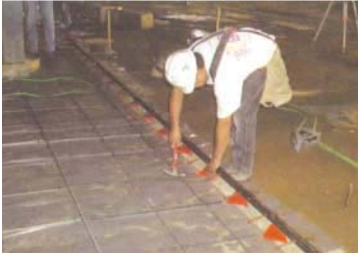
Left: the plate dowel pocket former is nailed to the form prior to casting the first slab.
