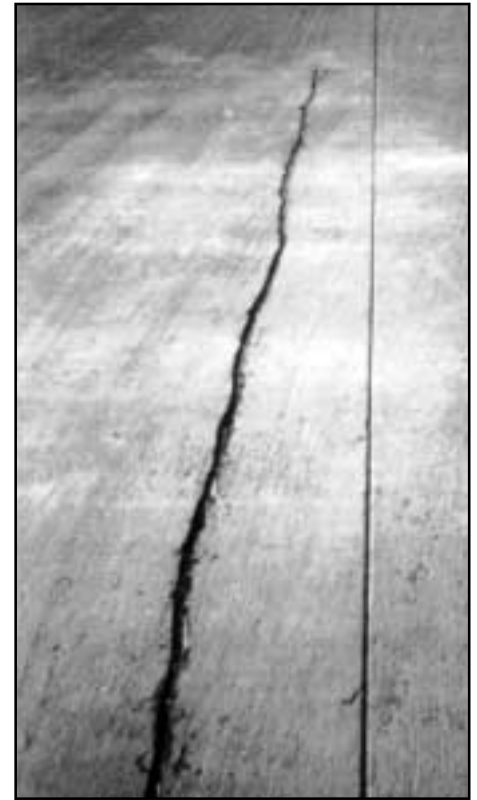
Crack due to misaligned dowel bars in a joint that opened. (Crack has been routed and sealed).
