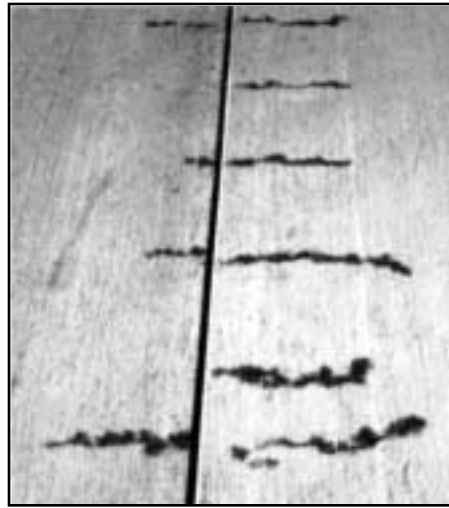
Cracks between dowels caused by their restraint of shrinkage parallel to the joint. (Cracks have been epoxy-injected).
